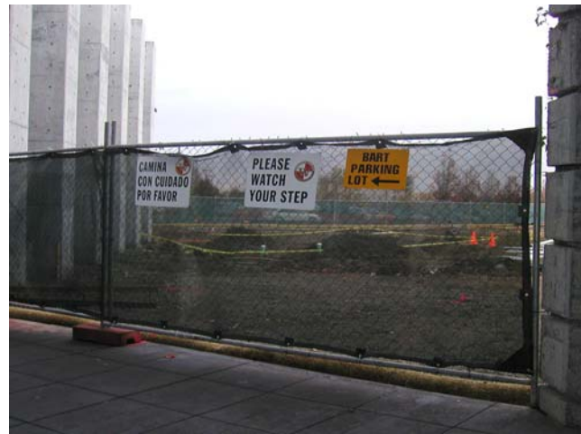
18. New parking structure construction site on north side of station adjacent to the existing parking lot and bus platform.
