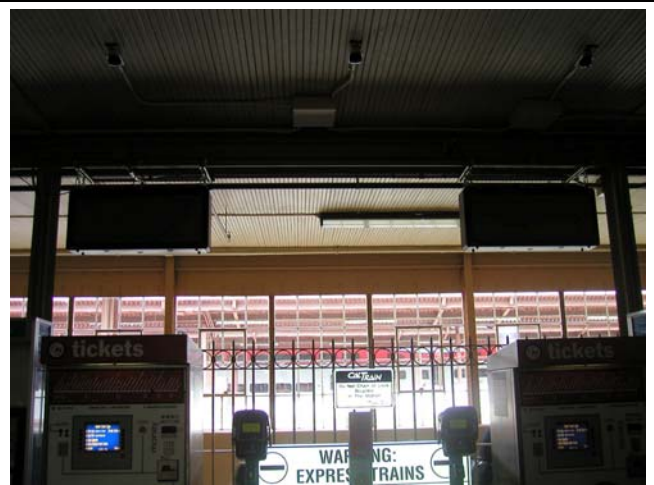
24. Non-operational Caltrain real-time signage
