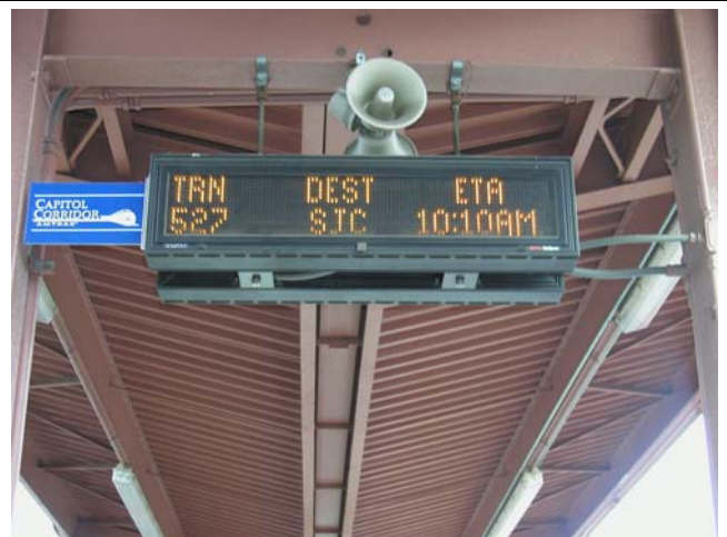
26. Capitol Corridor real-time signage on platform
