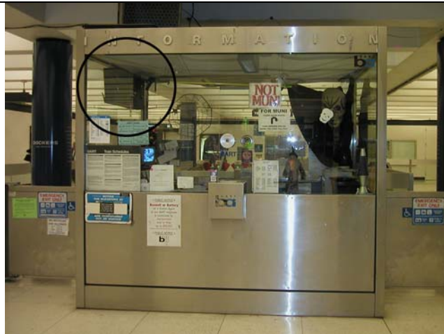
35. BART station agent booth. The variable message sign (circled) can be converted to next train information. This sign currently gives date, time and elevator status of the system.
