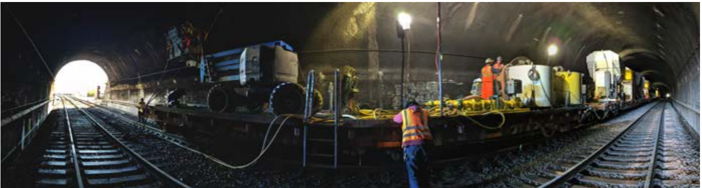
Construction of electrification infrastructure within rail tunnels in San Francisco (photo: Caltrain)
