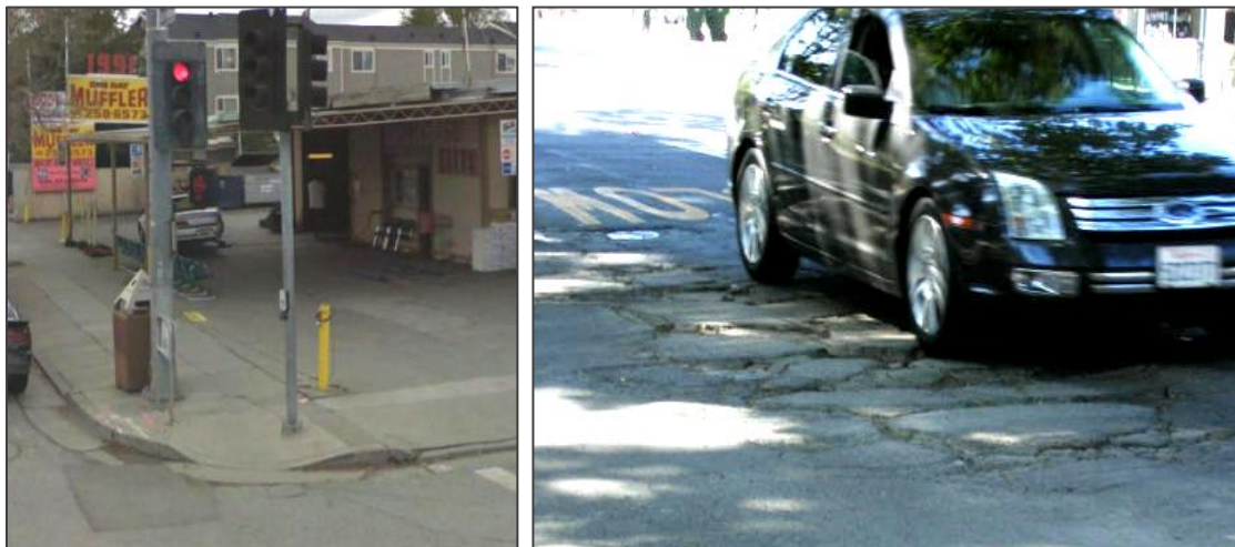
Figure 25 Deficient ADA Ramp on Alum Rock Ave. and Pavement Deterioration Along The Alameda in San Jose (Formerly SR 82)
