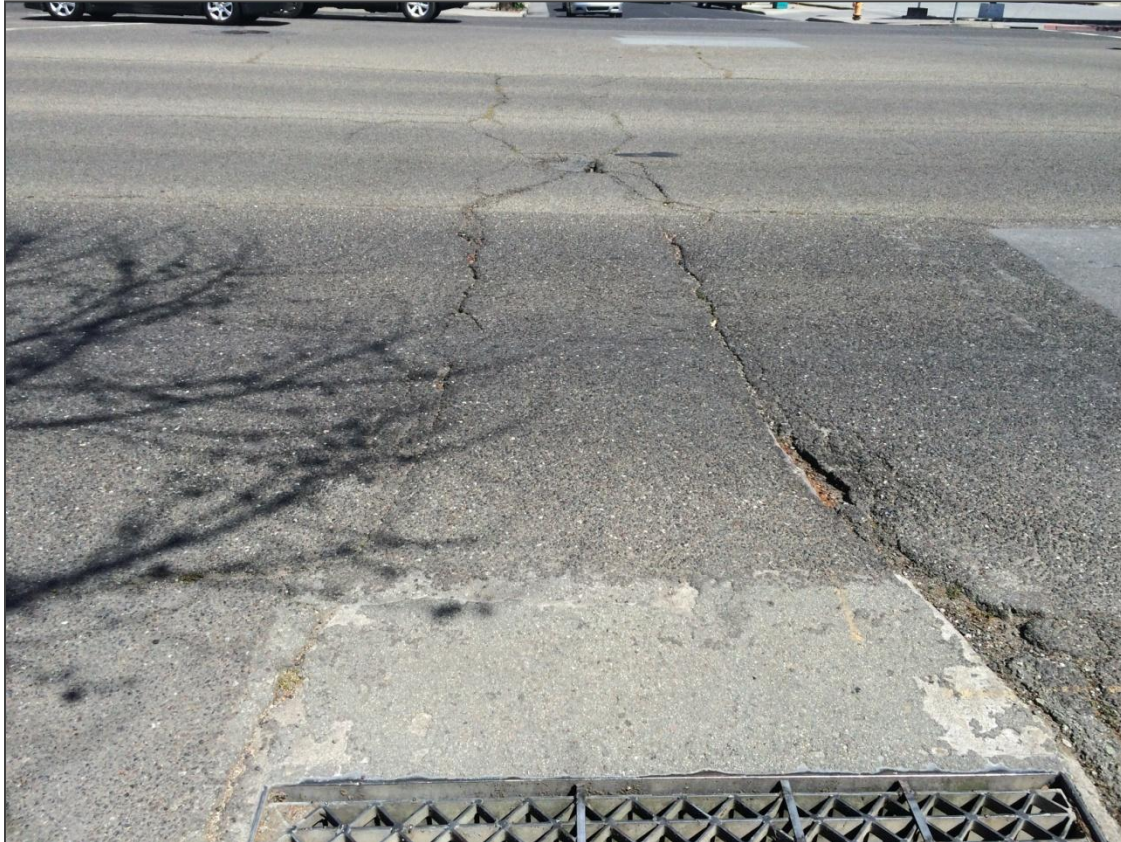
Figure 97 Pavement Exhibiting Signs of Possible Structural Distress on El Camino Real in Palo Alto
