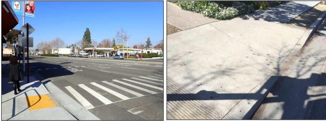
Figure 104 A Newly Installed ADA-Compliant Curb Ramp (Left) and a Curb Ramp Requiring Replacement (Right) on El Camino Real in the Study Area
