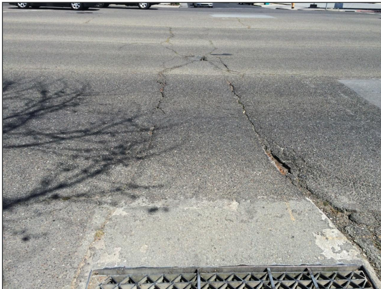
Figure 5 Pavement Exhibiting Signs of Possible Structural Distress on El Camino Real in Palo Alto
